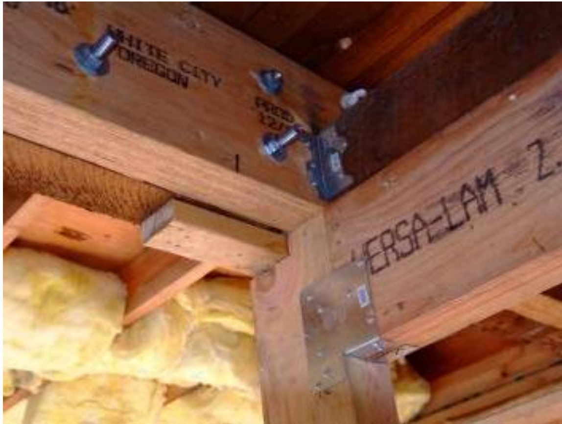
Napa, CA, Feb. 14, 2006 -- A homeowner retro-fitted their home with earthquake straps and bolts to prevent movement in the event of an earthquake. Photo by Adam DuBrowa.
