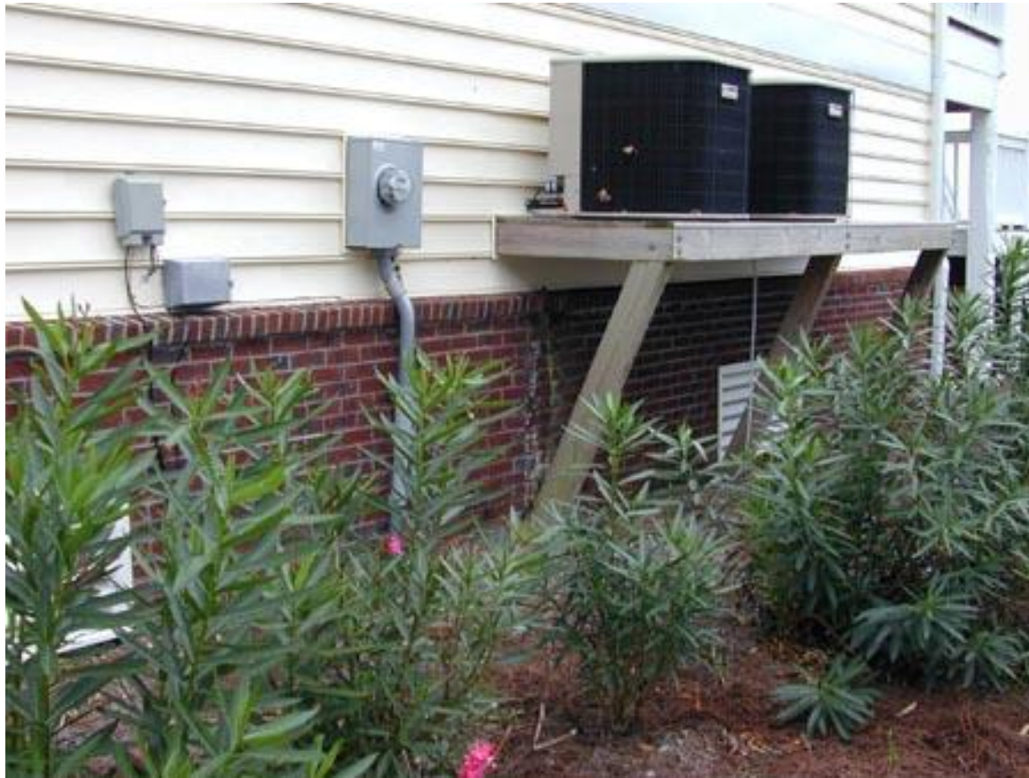
New Bern, NC. -- Southport, NC. – Elevated utilities offer protection from flooding and high water. Photo by Dave Saville/FEMA News Photo
