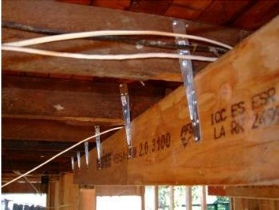
Napa, CA, Feb. 14, 2006 -- Earthquake straps hold this structure firmly to the foundation to prevent movement in the event of an earthquake. Photo by Adam DuBrowa.
